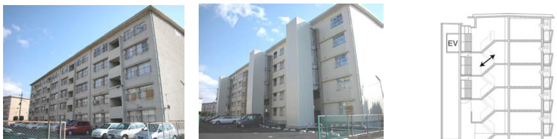
Figure 1. Building before and after the renovation work involving the addition of elevator towers, and section view
